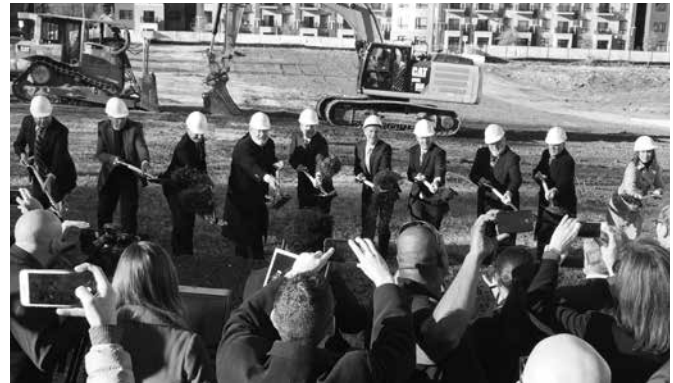
State leaders broke ground for the new State Library on December 11, 2017. Photo by Susie Webb Ries
